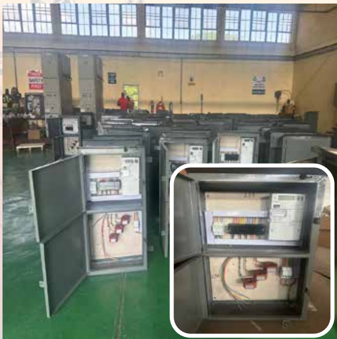
Wired single door smart metering cubicles
